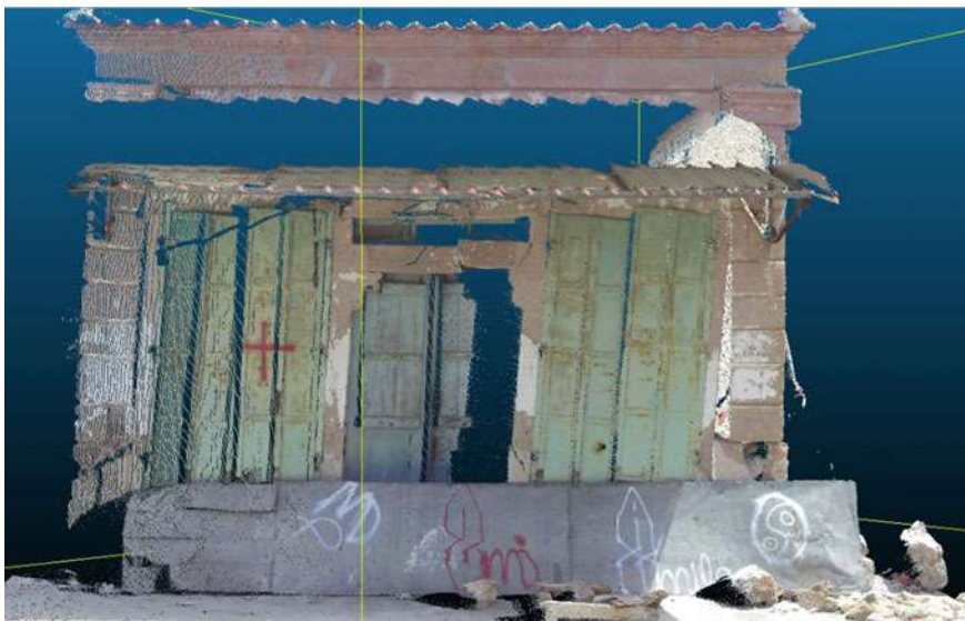
Fig. 17 An example from the third page of the proposed documentation of building damage assessment, which contains the 3D point cloud derived by TLS. The 3D measuring tool permits the accurate measurement of distances, angles and volumes
