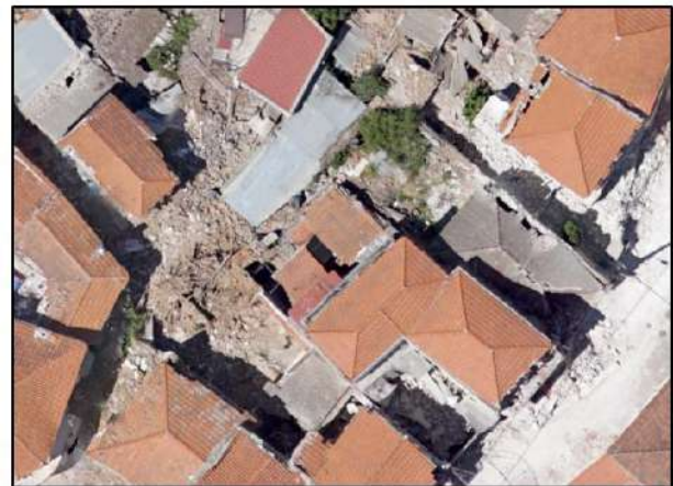
Figure 6. Part of the 13 th June 2017 orthophoto map at a scale of 1:500 with damages of grade 4 e.g. heavy structural failure of roofs and floors.
